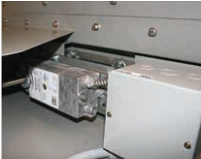
Isolation Damper Actuator and Transformer
