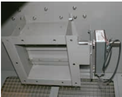
Bypass Damper Actuator
