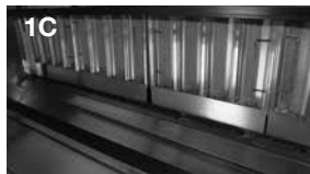
Grease Grabber™ filters, second row of filters
