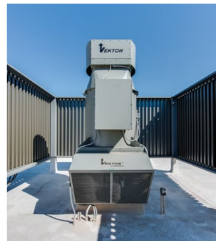
One of three Greenheck Vektor-HS fans installed to safely expel exhaust fumes from laboratories.
