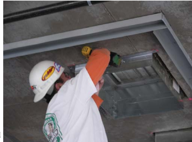
Brody Demoe of Doody Mechanical installing Greenheck dampers. The factory-installed convenience feature saves 52 minutes of installation time per damper.
