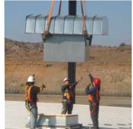
One of five hooded propeller fans being set in place on a roof curb.
