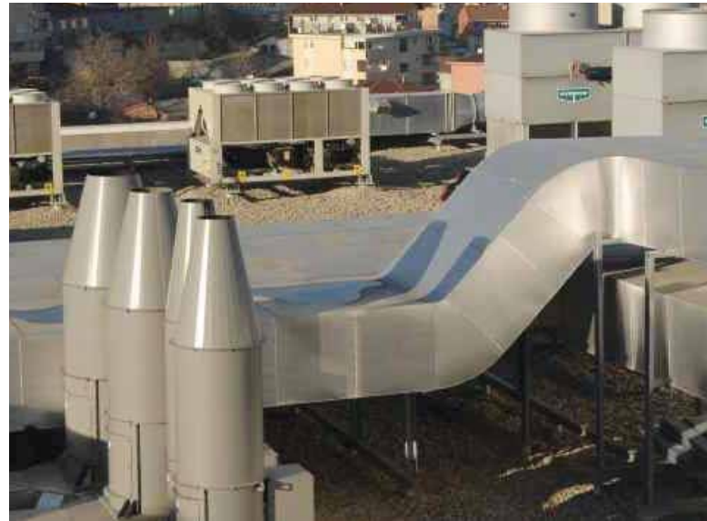
Above - Greenheck's Vektor-H laboratory exhaust units. A total of six units were used for kitchen exhaust.
