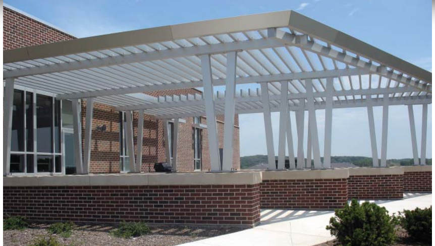
The custom sun control offers protection from the sun for resident firefighters and the public in this outdoor gathering area.
