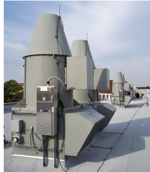
Three Vektor-H laboratory exhaust systems replaced 13 lab and general exhaust systems, resulting in decreased maintenance time.
