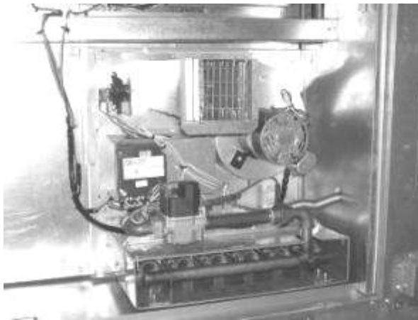
Figure 46 - Gas Heat Exchanger
