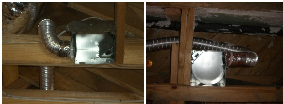
Figure 1. Common Installation Issues: Immediate bends after exhaust fan and 180° turns due to poor planning during installation.
