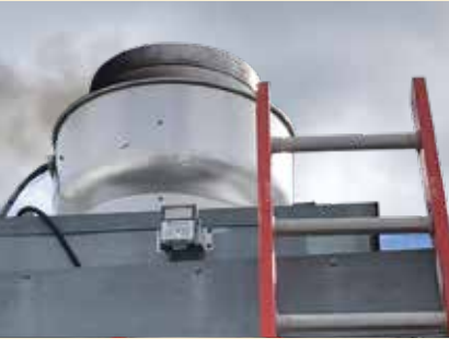
Model CUBE with a Vari-Green drive exhausting air during the abnormal flare-up test in accordance with the UL-762 certification.
