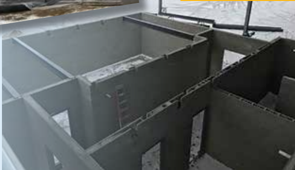
The roof is on at the National Distribution Center and ready for wall sections.
